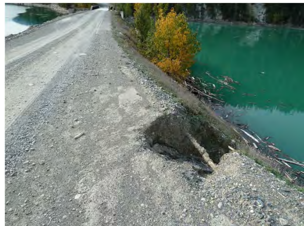
Figure 1-6: Bank erosion on camp end approach.
