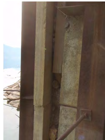
Figure 1-18: Woods end upstream wing wall gap.
