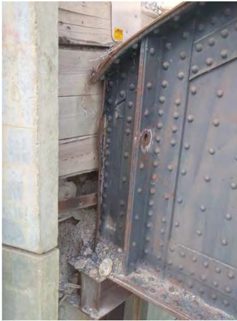
Figure 1-19: Woods end upstream planks missing.
